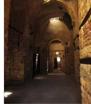
Ceiling and lighting system in the corridors (Saad, 2021)
