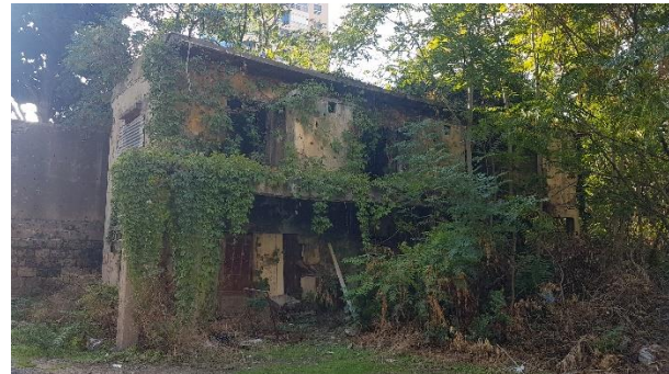
Figure 3. Nature recovers a war-damaged building along the demarcation line – Photo Credit: by Author – Jan. 2020.
