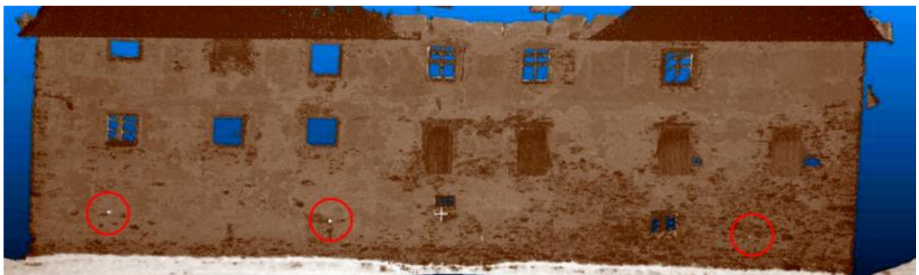
Figure 14. Raw scan of the west façade; the red circles mark the reflectors attached to the wall for georeferencing and comparison with the other partial scans
