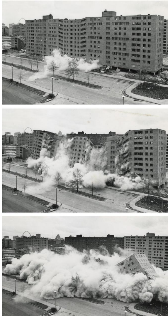
Figure 4. Minoru Yamasaki, public housing complex Pruitt-Igoe, St. Louis. Constructed in (1951-1955) was demolished in 1972-1976 (Source: U.S. Department of Housing and Urban Development)
